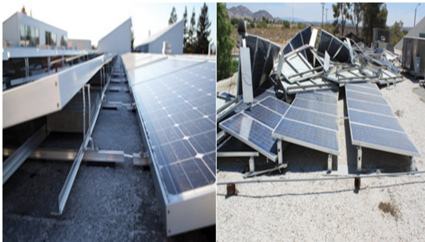
Figure 5. Failure and damage of the mount ground solar tracker caused by strong wind [37]
