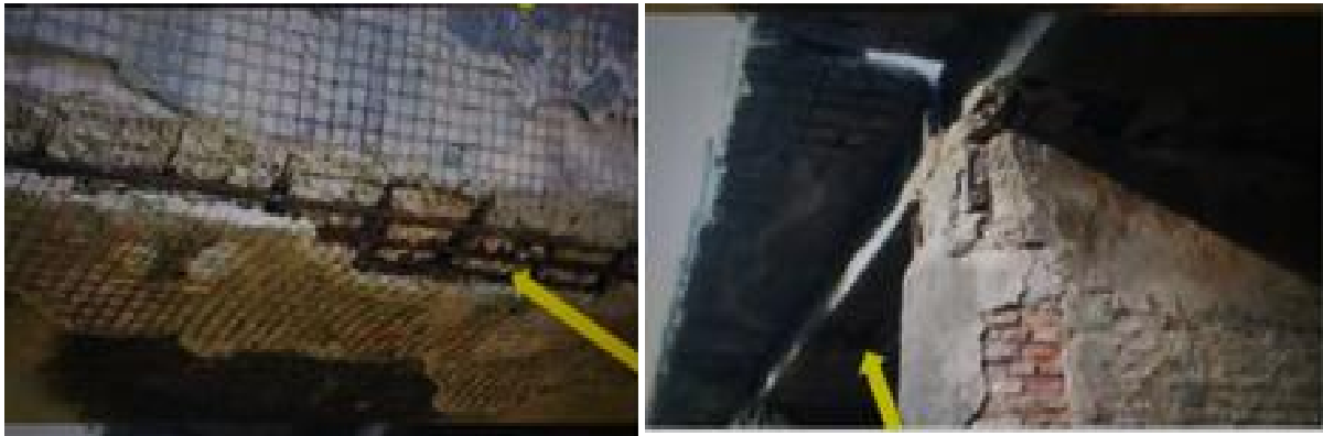
Figure 7. Concrete degradation of the bridge due to continued exposure to flood hazard.
