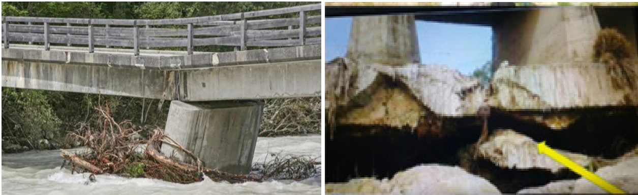
Figure 2. Bridge damage due to flooding hazard.
