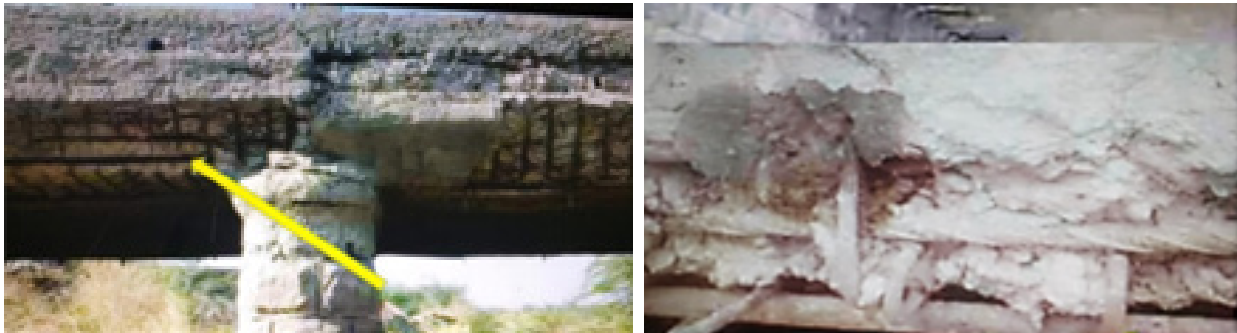
Figure 3. Bridge damage due to seismic hazard in the corrosion-prone bridge.
