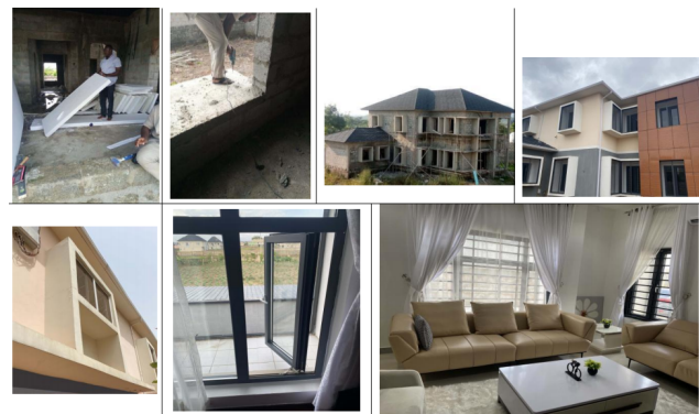
Figure 8. Pictures of different stages of construction of finished MSS in a typical residential house (Source: author's project).
