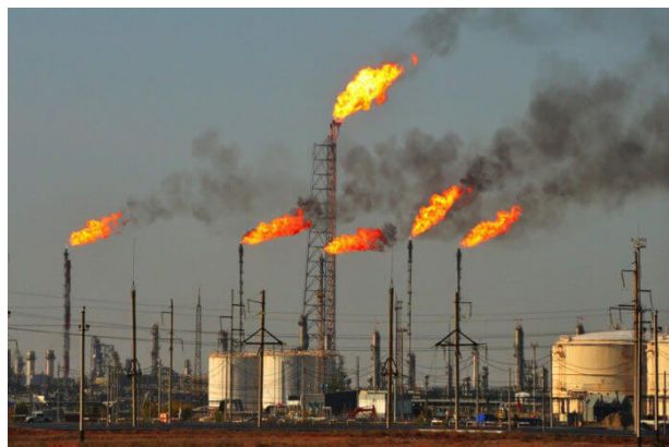
Figure 1. Gas flaring site [12] .
