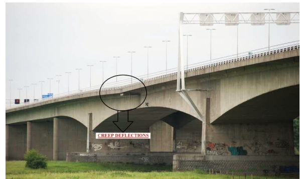
Figure 8. Creep-Induced Mid-Span Deflection in the Alvik Bridge, Sweden [109] .
