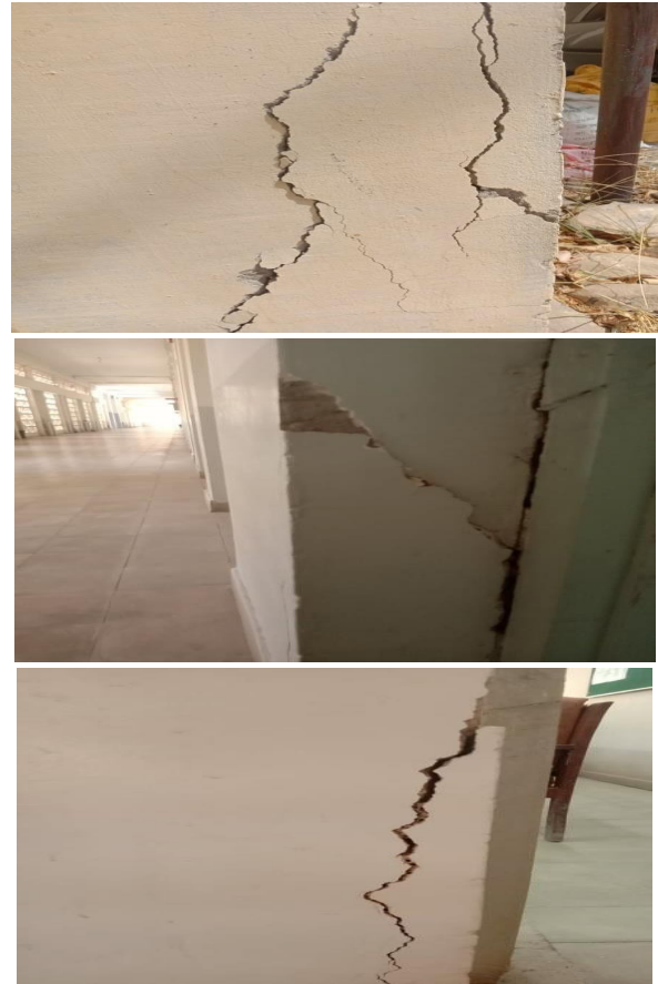
Figure 2. Cracks showing size and orientations in the building
