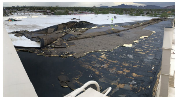
Figure 10. Roof “B” After Storm
