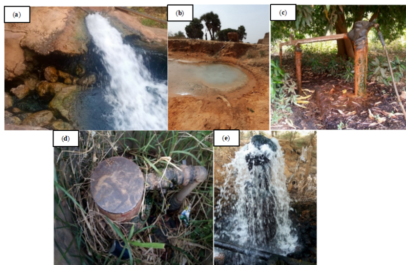
Figure 7. Damaged technical equipment: (a) Drill head torn off by artesian pressure at Koutoumbou; (b) PVC casing and wellhead expelled by overpressure at Garin Kio; (c) Corroded drill head equipment at Yélou; (d) Flooded drill head at Timba; (e) Spontaneous and diffuse outflows on the Dioundiou 1 borehole.
