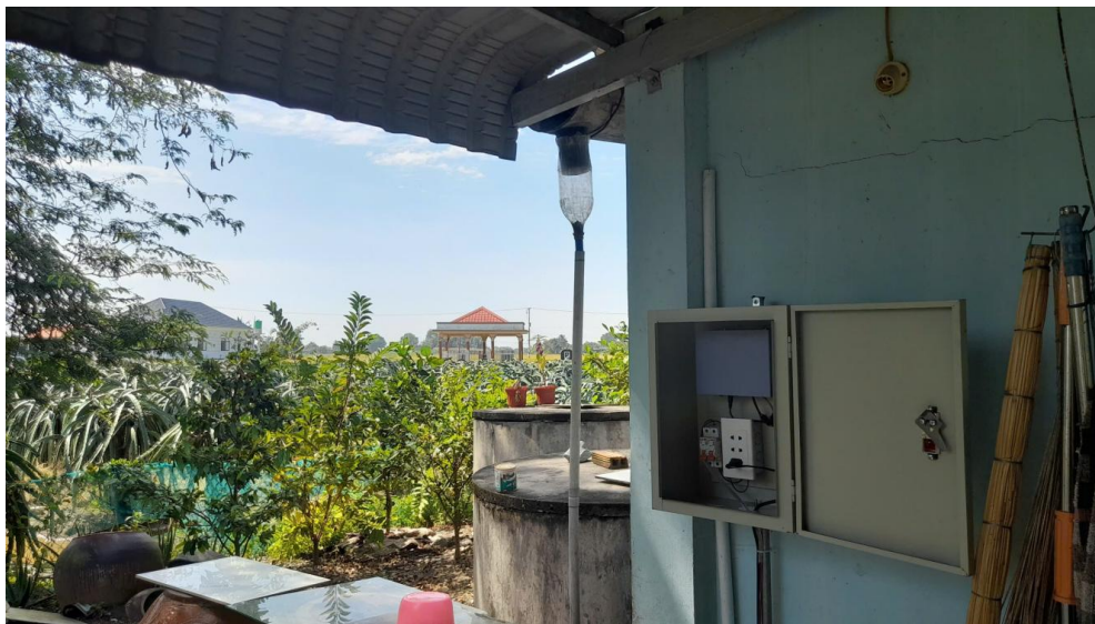
Figure 8. An electrical cabinet containing the microprocessor of the IoT system.
