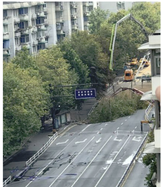
Figure 2. The construction accident of Hangzhou Metro Line 5, China
