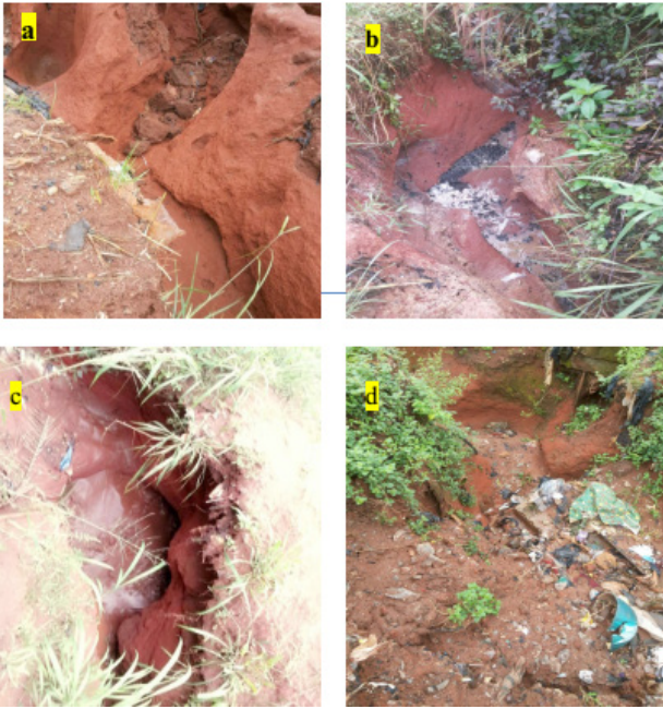
Figure 2a, b, c and d: Shows erosion sites at Old Abraka road-Boji Boji Owa-Ika North-East, Power Line road-Boji Boji Owa-Ika North East, Baleke street Boji-Boji Owa- Ika South and Doctor White Boji-Boji Owa-Ika South respectively.
